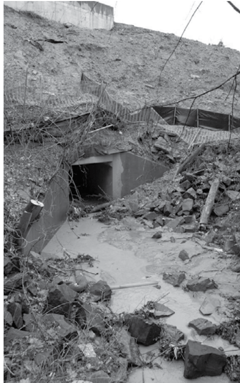
Polluted water is leaving the HOT Lanes construction site and entering Accotink Creek. Photo by Kris Unger.
